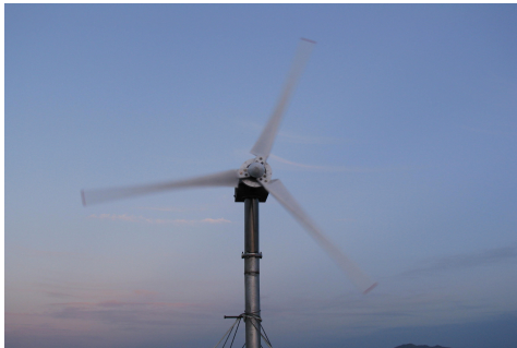
Fig. 28 Operating wind turbine system.
